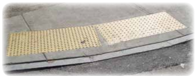
These truncated domes are not set correctly - they must span the curb cut width.
